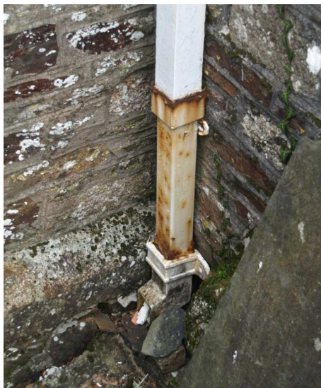
Downpipe at west end of south aisle showing corrosion and section of pipe of wrong size.
