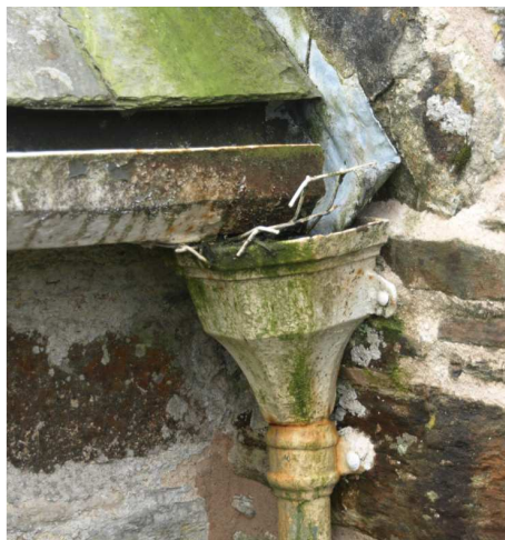
Top of downpipe on the west side of the vestry, showing evidence of corrosion and water overflow. The pipe here is too small as it takes a large proportion of the water from the nave roof as well as the vestry. It needs a larger cast iron hopper and wider square profile downpipe.
