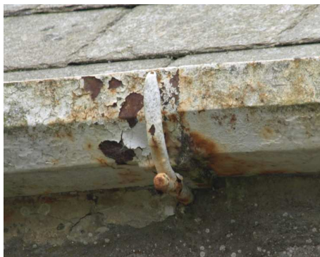
Corroded joint with two sections out of line and with corroded back face to the gutter.
