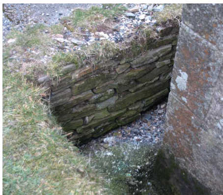
The trench that surrounds the church is the only means of draining water away. This part of the trench side at the south east corner had to be rebuilt recently because of damage caused by water flowing out of an open gutter end.
