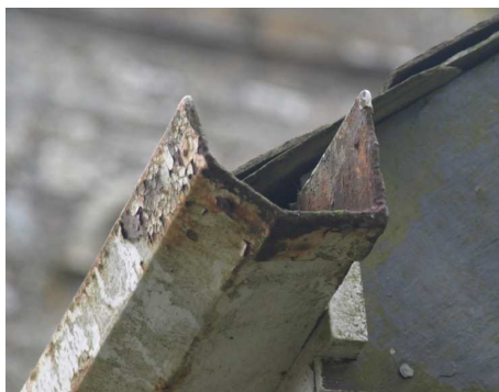
One of a number of missing gutter ends.
